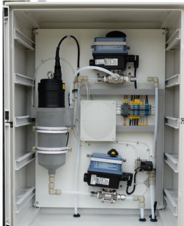
Water sampling container with vacuum pump. Auxiliary clean water supply
