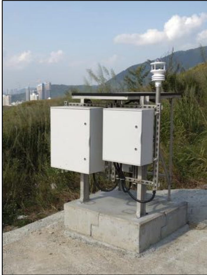
Autonomous monitoring station running on solar power
