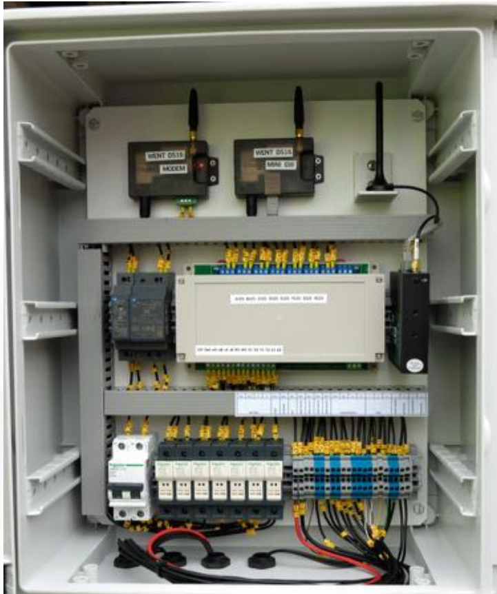
Control panel with Synap wireless equipment and 4G modem
