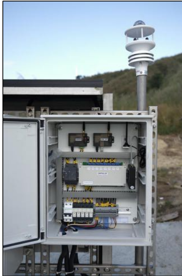
Control panel with Synap wireless equipment and 4G modem
